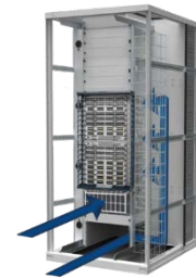
Switching and Routing Racks
